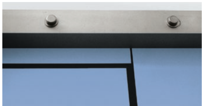
SUPPORT AREA FOR INWARDS OPENING DOORS A MINIMUM OF 80 MM HIGH, IN ORDER TO BE ABLE TO HANG THE DOOR, DIMENSION A.
